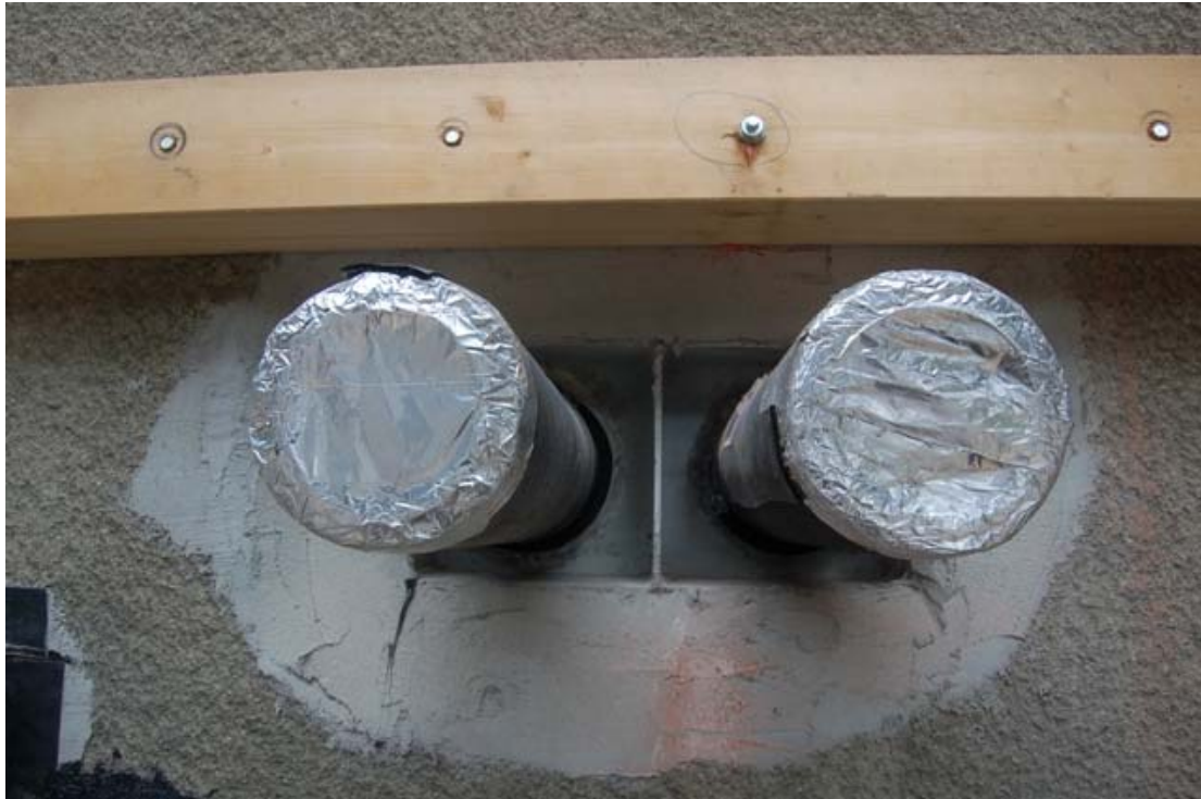
Picture 4.8: Outlet and inlet pipes at reconstructed house in Frankfurt (Germany).
