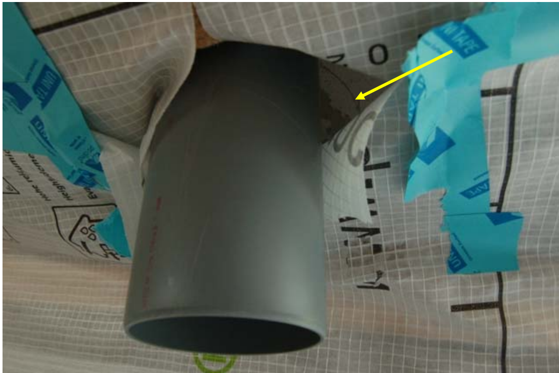
Picture 5.3 (e.u.z, Germany 2009): Demonstration of improper insulation lowering air tightness of a building and energy losses.
