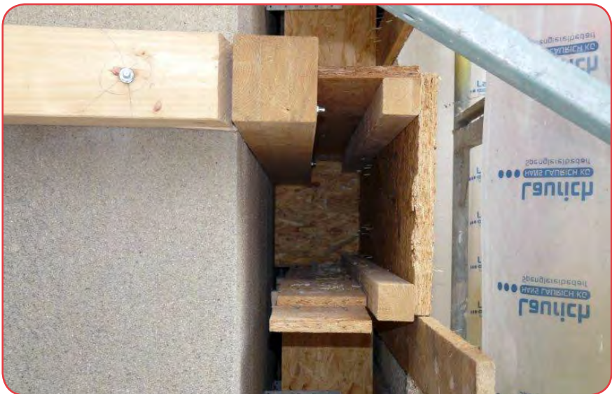
Fig. 5. Prepared wood casing on an outside wall to be later filled with insulation material | Image: © Jörg Faltn
