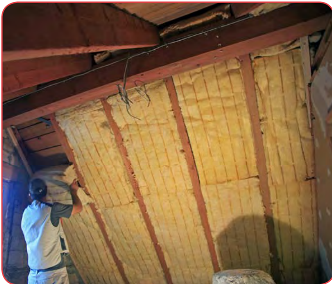
Fig. 6. Adding of rafter insulation to decrease the heat loss through the roof. Image: © Rainer Sturm | PIXELIO.
