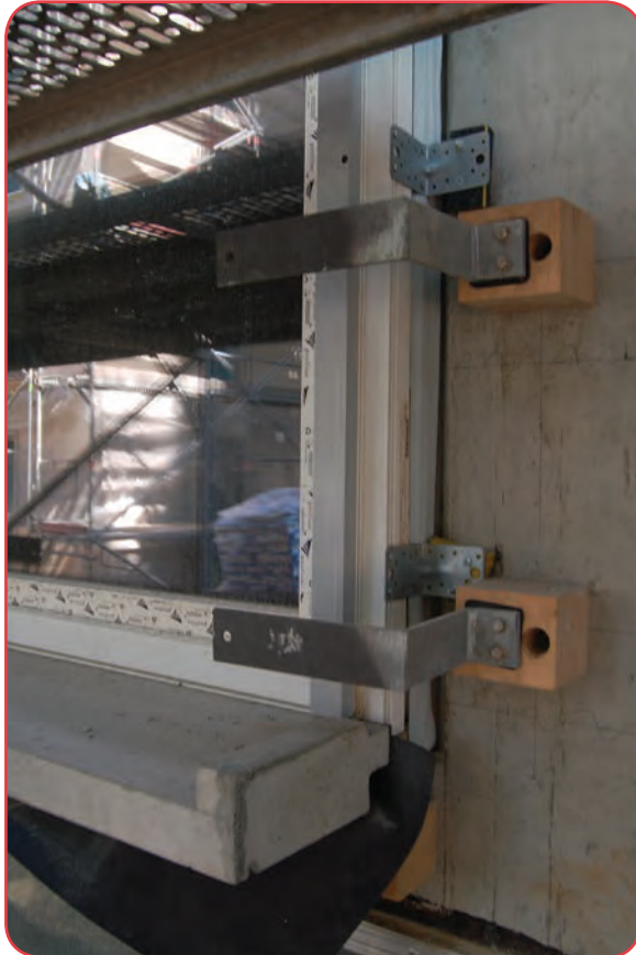
Fig. 2. Avoiding thermal bridges during construction accounts for a large part of the later saving potential of the building. | Image: © M. Tvrdoň
