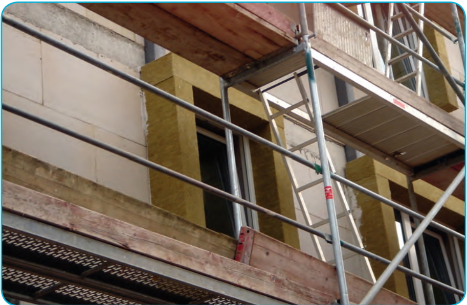
Fig. 3. 30 cm of insulation being installed at a passive house. | Image: C. von Knorre
