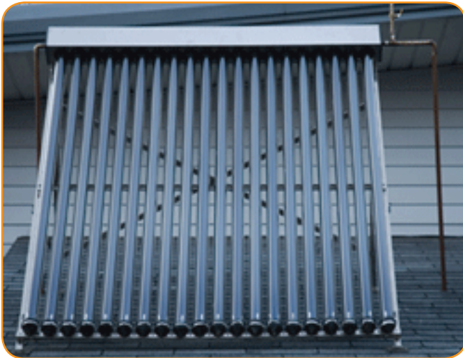
Fig. 2. Example of solar panel for water heating
