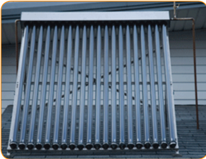
Fig. 2. Example of solar panel for water heating
